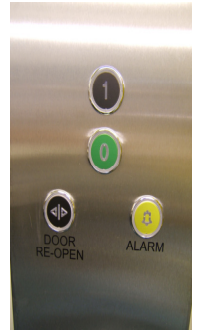
Cabin control panel
